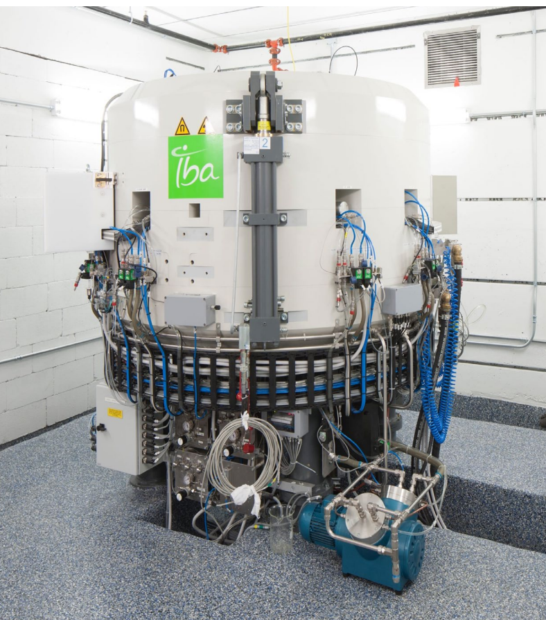
The Cyclotron in its vault
